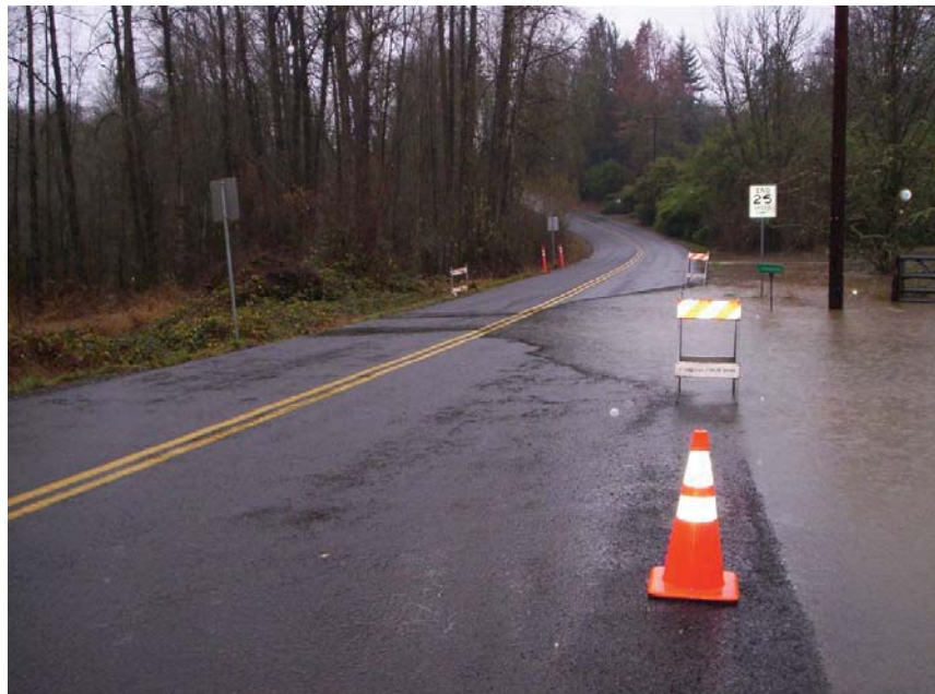
Undersized culvert causing overtopping of roadway during heavy rains (multiple times per year)
