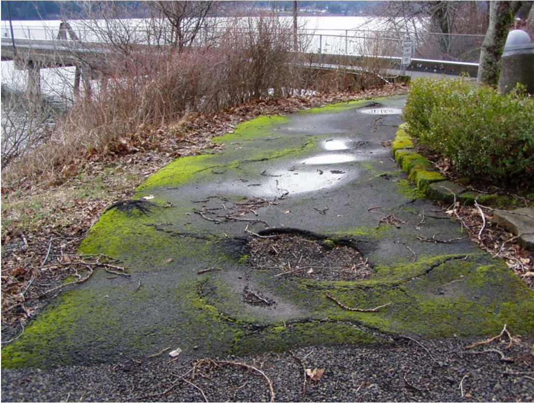
Current Trail with Erosion Damage
