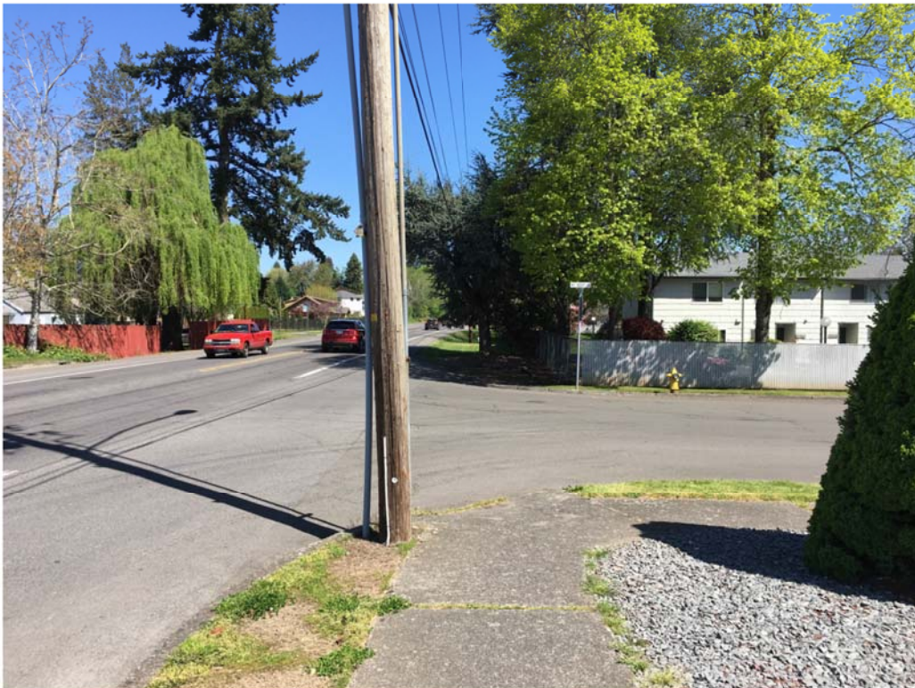
Intermittent sidewalk ends and curb ramps non-compliant/missing.
