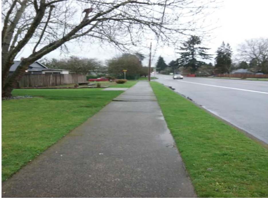
Existing damaged sidewalk to be replaced.
