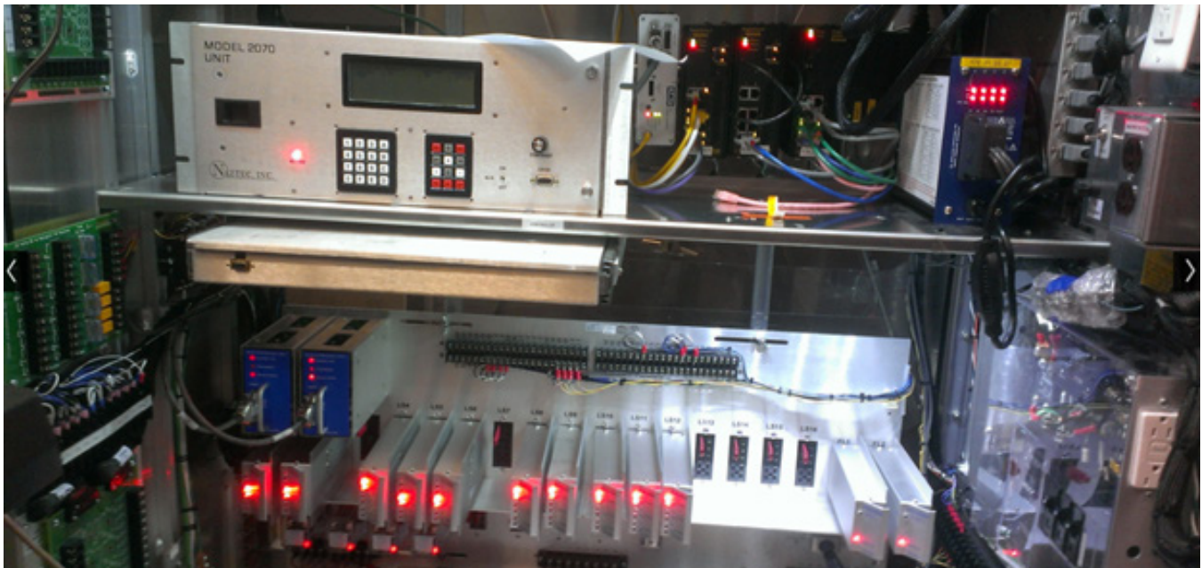
Figure 17: TSMO is supported by a network of ITS devices, communications, and data – key assets to be managed and replenished to ensure the effectiveness of the TSMO program.
